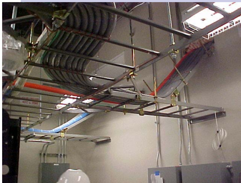
Copper & Fiber Risers
