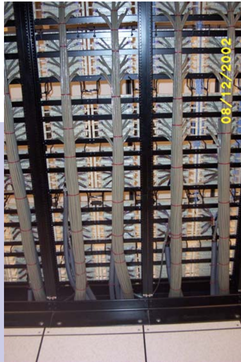
Rear View Voice Riser Dressing from below raised floor
