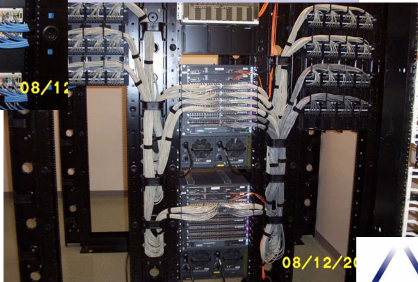
Patch Panel Front View
