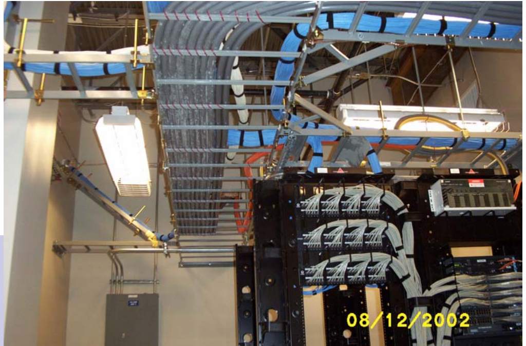
Ladder Rack View
